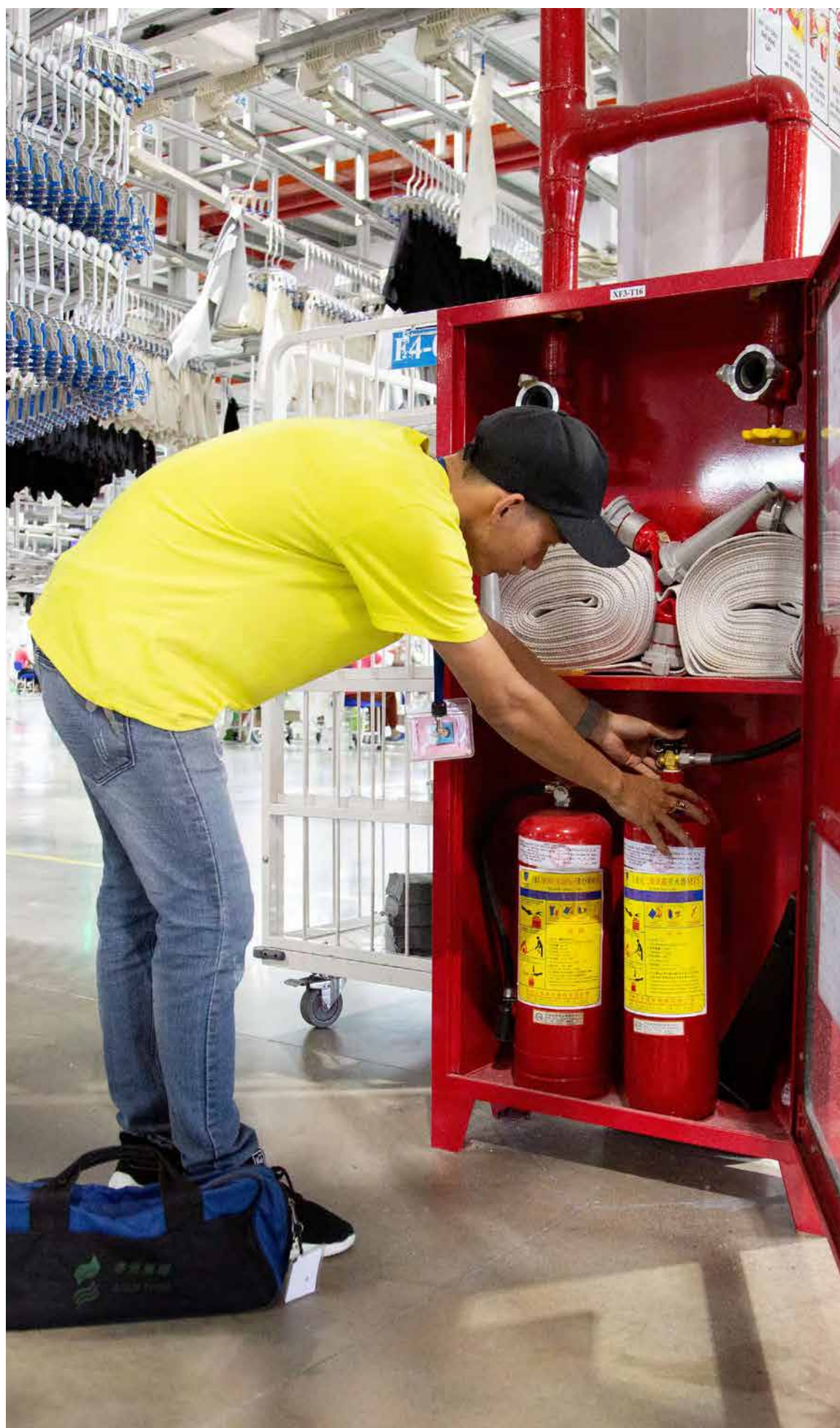
A teammate checks fire safety equipment at Shenzhou's Worldon apparel factory in Vietnam.
