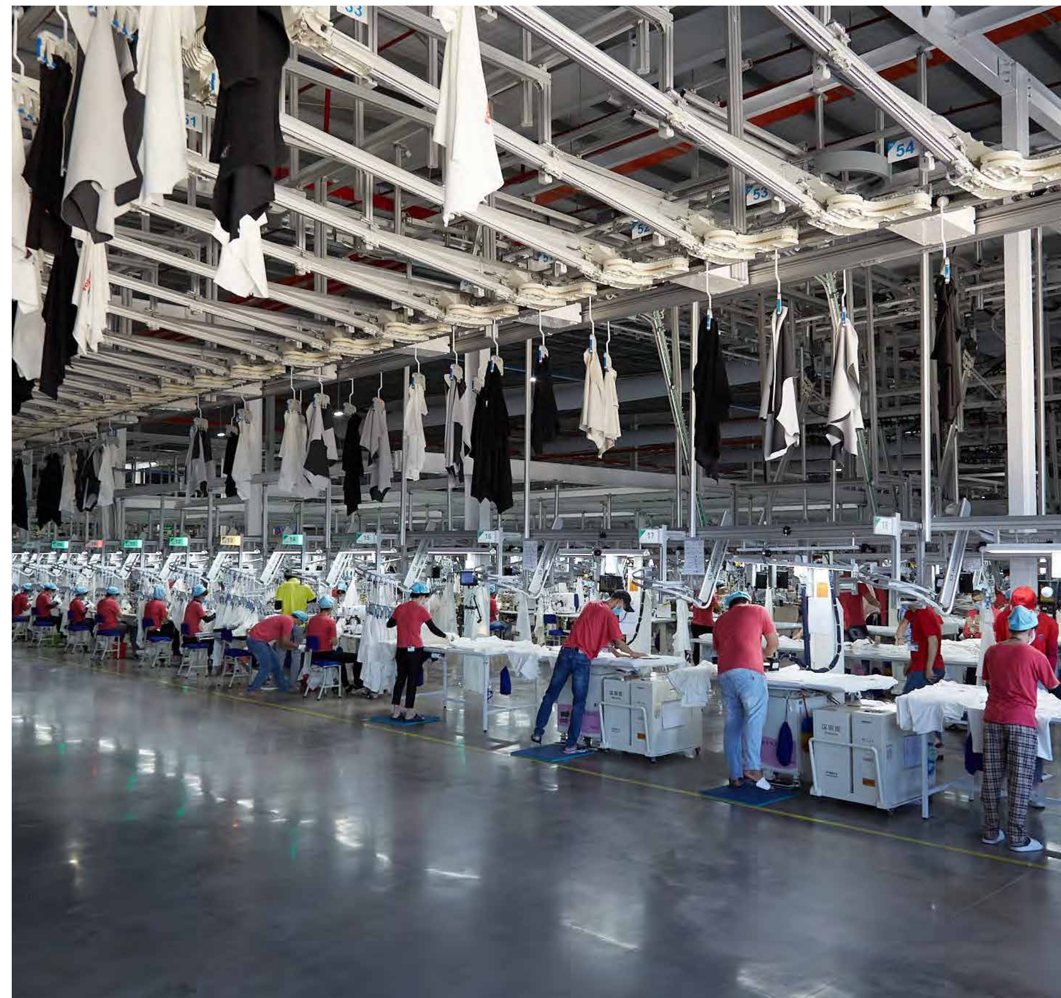
A Shenzhou facility in Vietnam has replaced a centralized coal-fired boiler system with electric boilers, greatly reducing GHG emissions.
